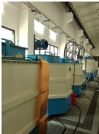
120kV serial resonant high voltage power supply
